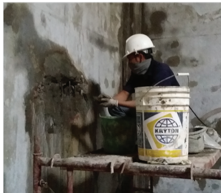
A LEECON Ltd, applicator applies the Krystol Crack Repair System to the damaged water tank.
