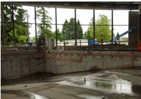
Looking at the deep end of the pool. The red lines is the Krystol Waterstop Grout used to waterproof the cold joints.
