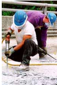
Do not skimp here. Its prep, prep, prep if the repair is to last.
